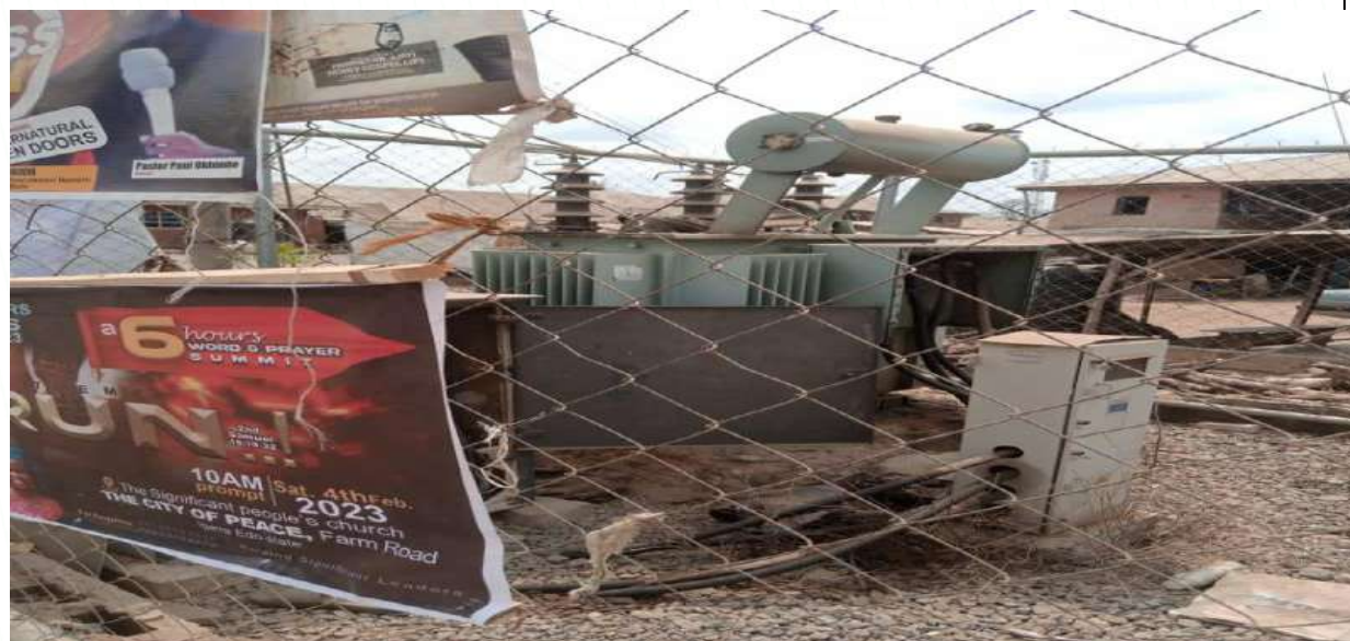
Transformer delivered to Ikpeshi community
