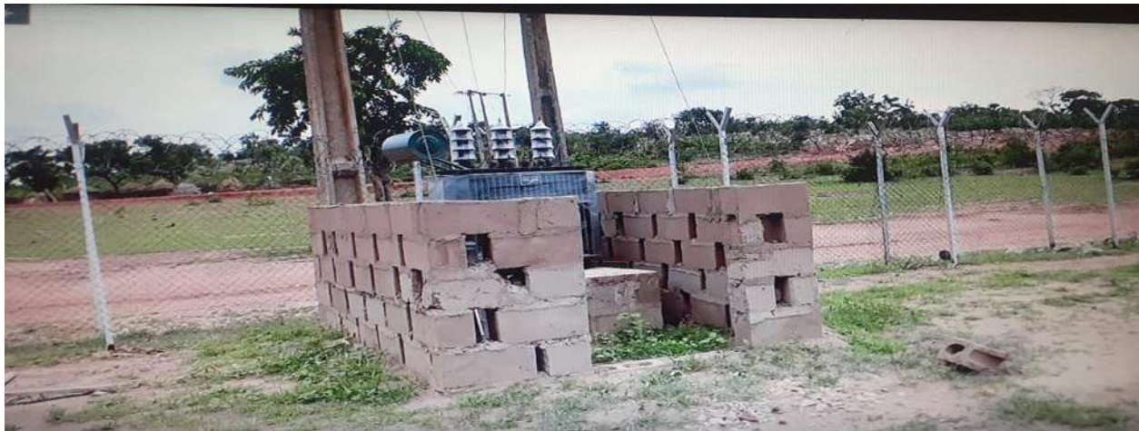
Figure 5:1 CDA Rural Electrification Project Executed by Yomed Nigeria Ltd in Kamtu, Kebbi State
