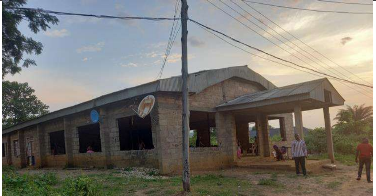
Abandoned Townhall project started in 2010 in Ikpeshi
